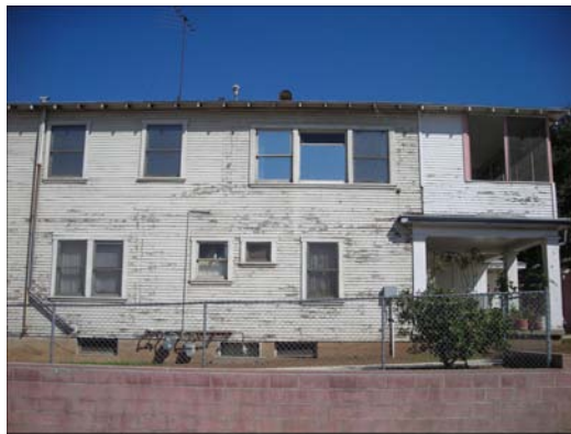
A home with LEAD contamination before CAPSBC work begins to eliminate the health hazard.
