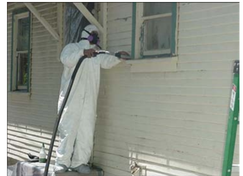
A CAPSBC LEAD removal technician carefully strips off the old LEAD based paint.
